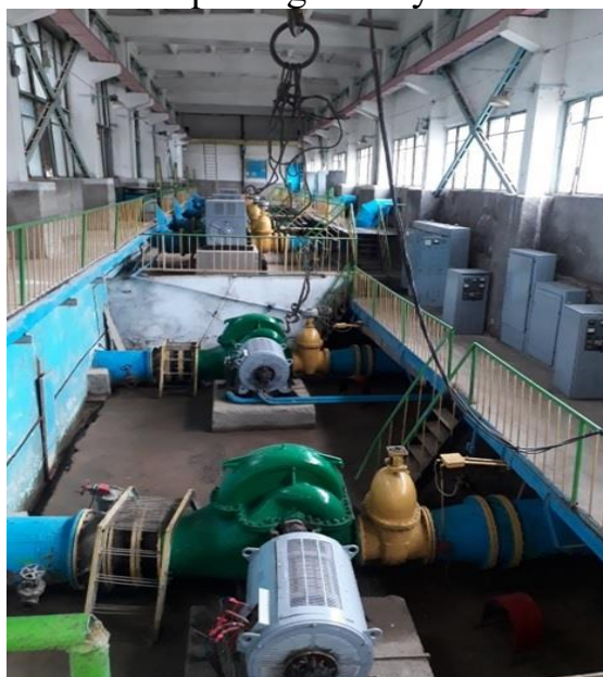
2-rasm. “Ramadan” nasos stansiyasining mashina zalining ko‘rinishi
